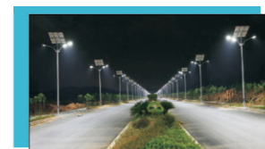
Street lighting system
