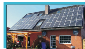
Off-grid home solar system
