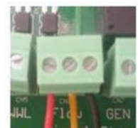
Flow Meter Terminal
