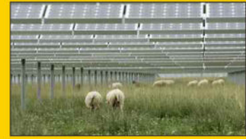
Farm solar generation system
